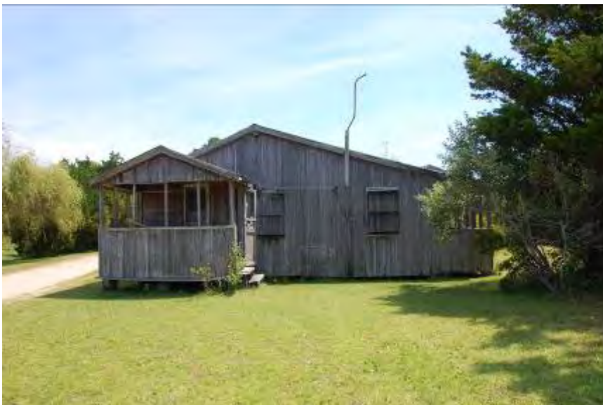
FIGURE 157. Overhead lighting on exterior of the Setzer-Dawsey residence is no longer functional.
