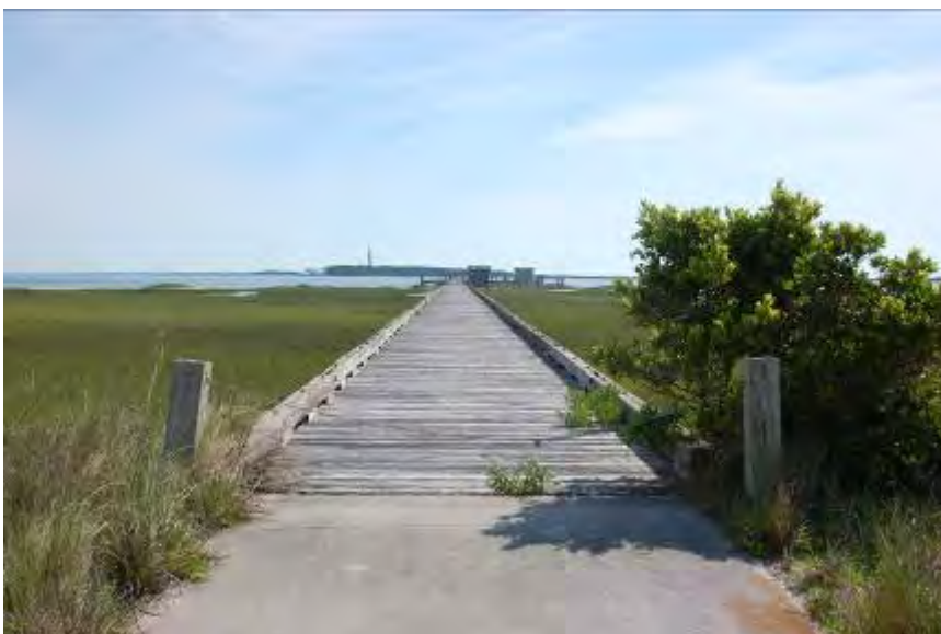
FIGURE 141. Wood ties along the sides of the Coast Guard Dock create raised edges.
