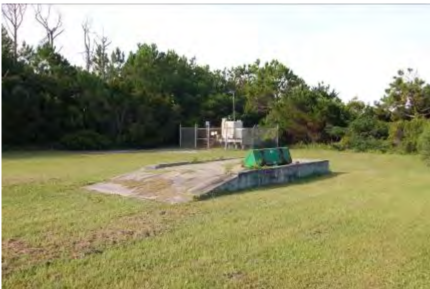
FIGURE 90. A concrete foundation with attached ramp is located south of the former Coast Guard Station garage.
