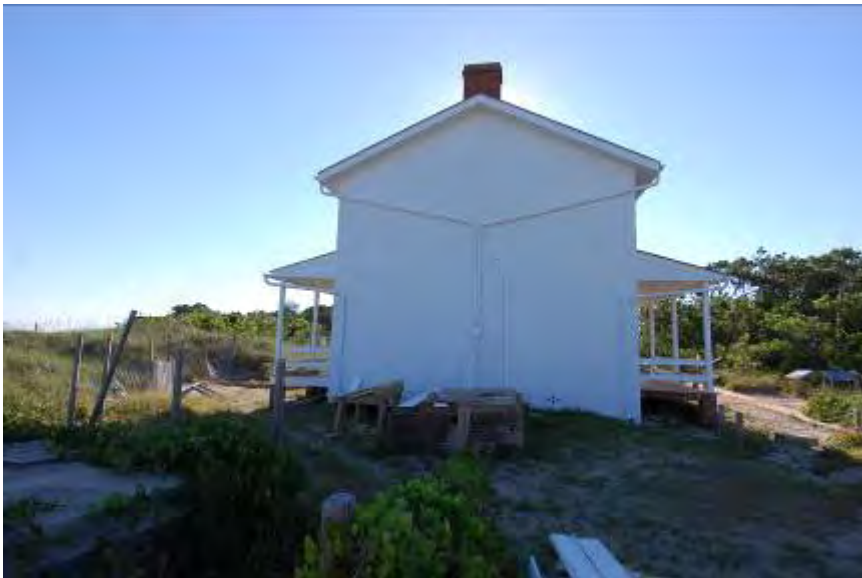
FIGURE 152. Wood posts on west side of the Keeper's Dwelling visible on left side.
