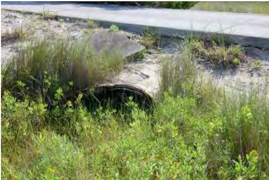
FIGURE 142. A metal culvert runs under the Concrete Road and helps drain an area that is subject to frequent flooding.
