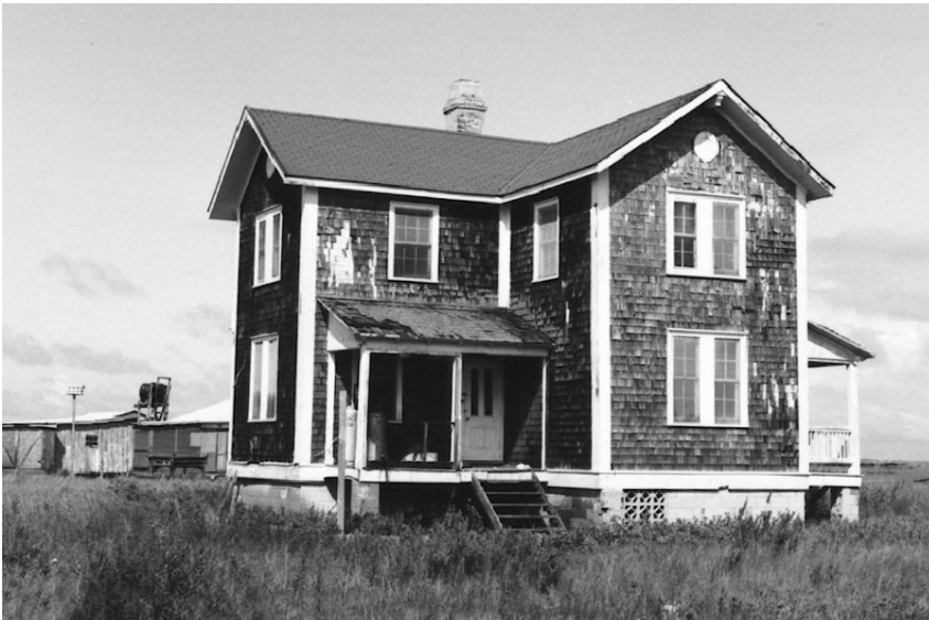
FIGURE 60. Side view of the Barden House (1907 Keeper's Dwelling after relocation), looking south, circa 1970s, showing rear porch.
