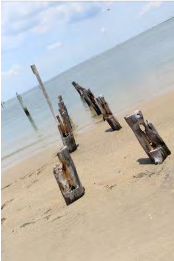
FIGURE 146. Remnant pilings of a former dock are evident near the bight end of the village.
