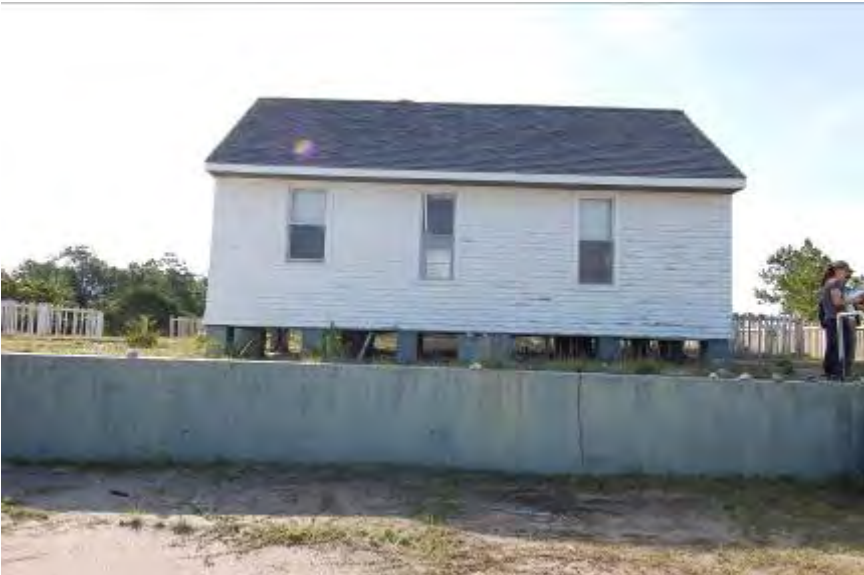
FIGURE 86. A concrete block retaining wall edges the parking area below the Coast Guard Station summer kitchen.
