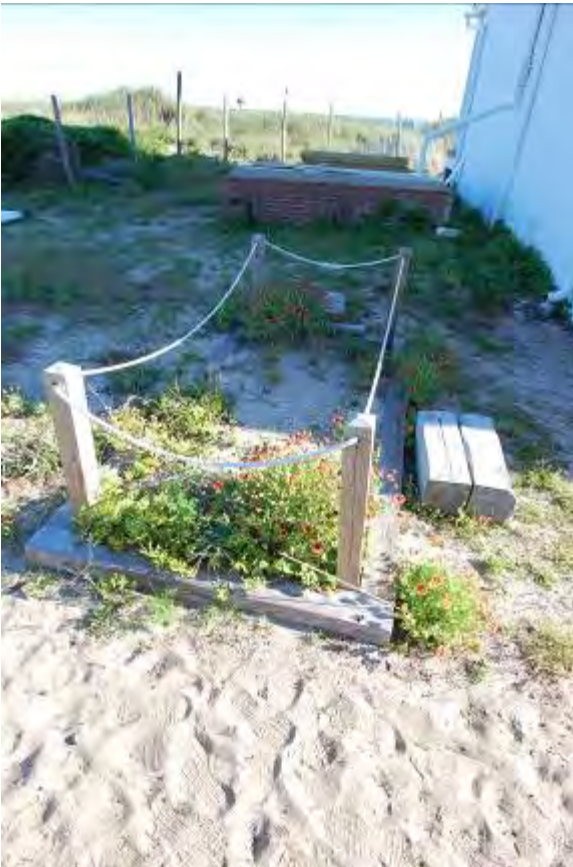
FIGURE 167. Wood-lined septic system located adjacent to the 1873 Keeper's Dwelling with cistern in background.
