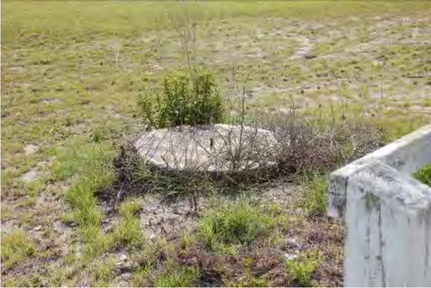
FIGURE 166. Additional water-related utility feature at the Coast Guard Station.
