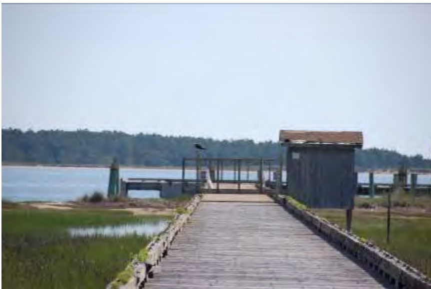
FIGURE 116. The Coast Guard dock is a concrete slab mounted on wooden pilings and edged by bolted timbers.
