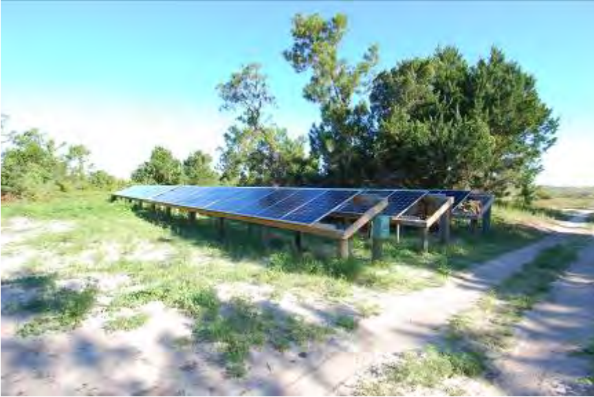
FIGURE 162. Solar array at the Lighthouse Complex, near the ATV shed.
