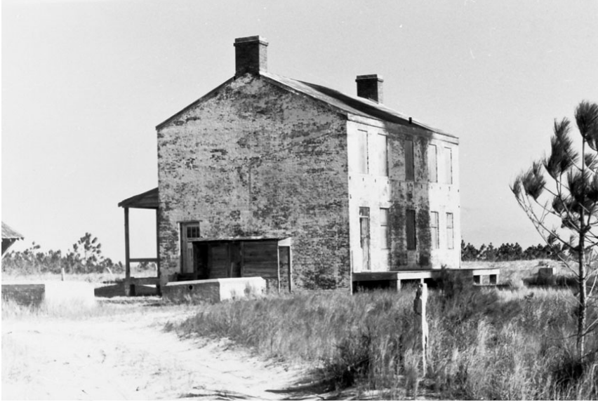
FIGURE 47. Lighthouse Keeper's Dwelling established in 1873, looking north, circa 1970. Note the outline where former downspouts were removed.
