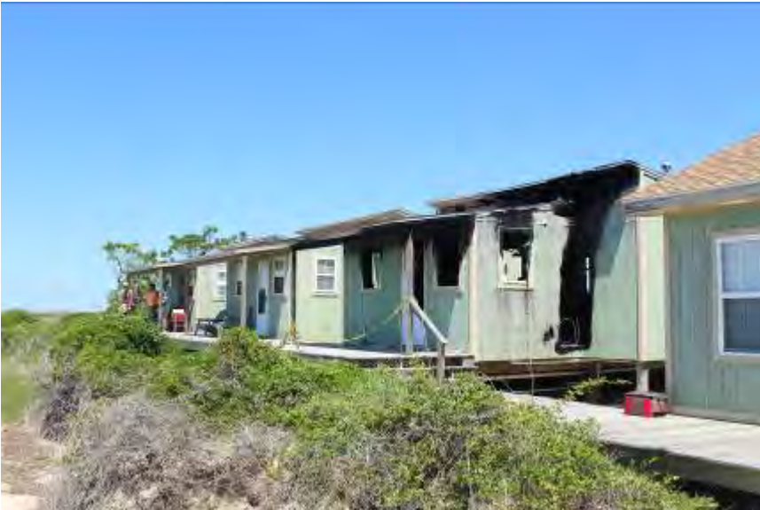
FIGURE 56. The three small rental cabins at the Les and Sally Moore Complex are identical wood frame buildings. The cabin closest to the Les and Sally Moore House (third from left) experienced a gas fire in 2016.
