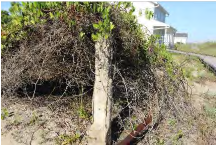
FIGURE 130. Concrete posts are remnants of a former fencing system that encircles the lighthouse precinct.
