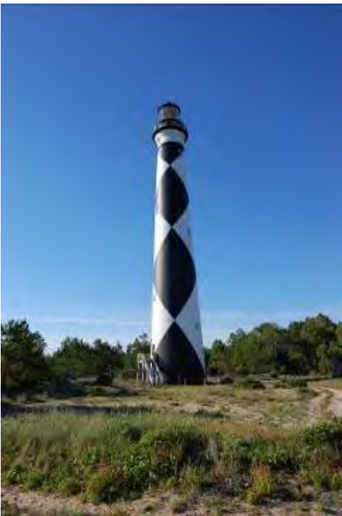
FIGURE 44. The Cape Lookout Lighthouse is a brick masonry structure painted with a black and white diagonal checker pattern.
